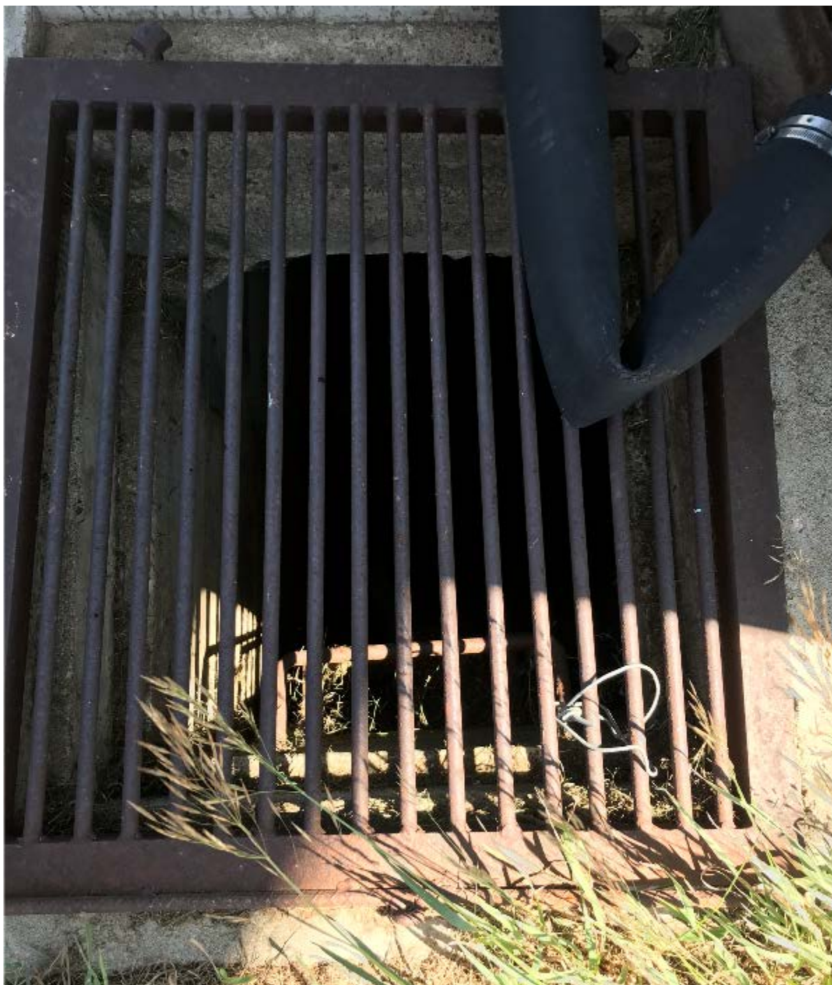
Image 4. 317 – 1 st Avenue, Tower Vault (2021)
