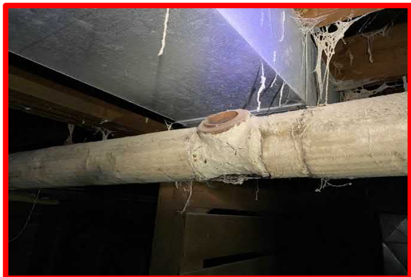
A1- Elbow Insulations/Basement
